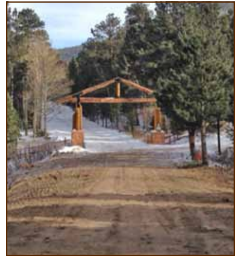
The main entrance to Land O' Peaks during and after the road repair process.
